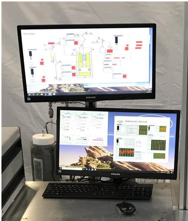
Dual-screen control station — synoptic + acquisition
